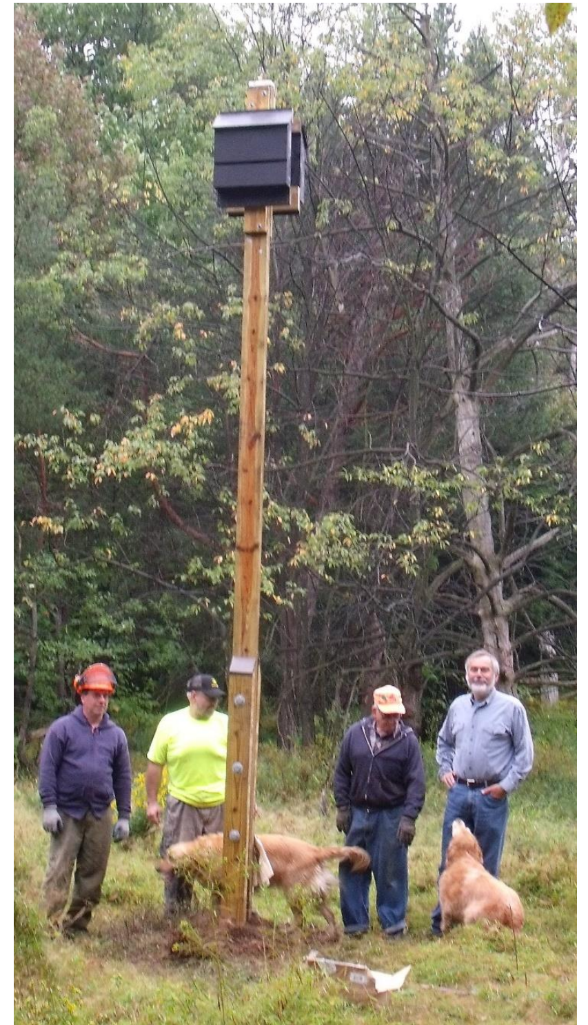
Above: A completed bat box at Beaverdam Sportsmen's Association – one of several that Adam (wearing safety helmet) has erected. Greg Gdula is on the far right and is Adam's right-hand man.
