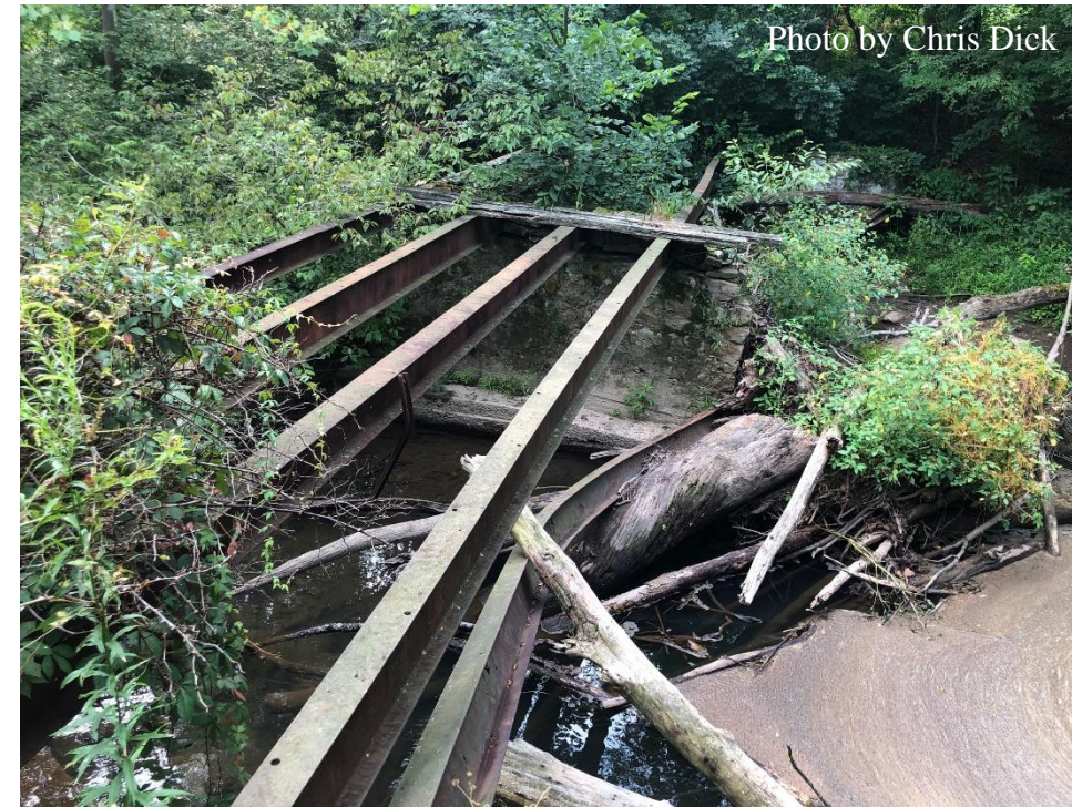
Remains of the Dunnings Creek bridge that once provided public access to the wetlands.
